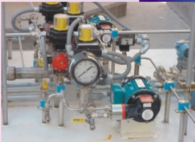
NOX Reduction Ammonia Injection
